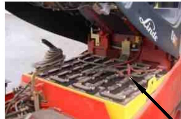
Fork Lift Batteries
